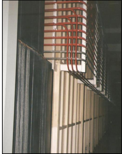
Paint Circulation Piping System for The Paint Shop
